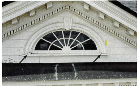
East Portico Gable: The gable window casing is deteriorated on either side where it intersects the sill (arrows). Gaps are present beneath the arched sash and the sill.
