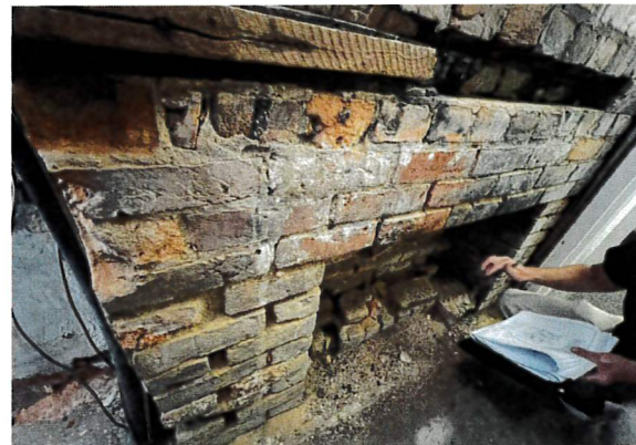
Lancaster County Courthouse: The fireplace has extensive mortar loss and settlement.
